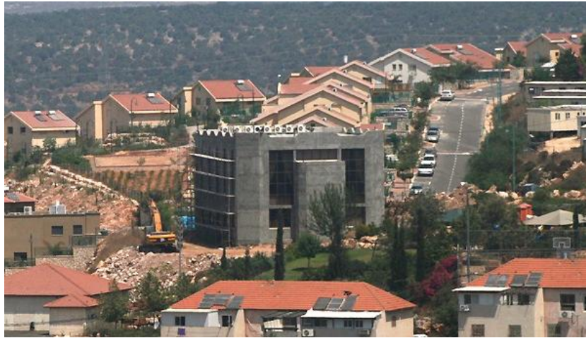
Revava (near Salfit) - Public building for religious purposes (synagogue or Jewish seminary) under construction. August 2010 – Al-Haq©
