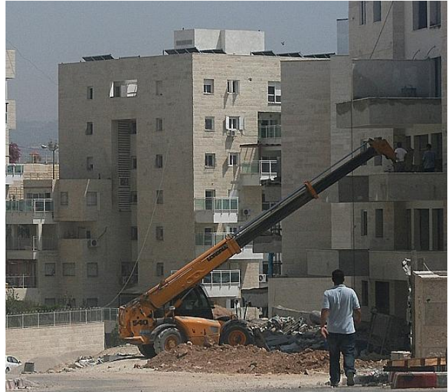
Modi'in Ilit – (near Ramallah) – Apartment buildings in final stage of construction. August 2010 – Al-Haq©
