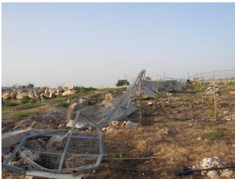
Figure 2: A retaining wall demolished in Khirbet Jubara, Tulkarem
