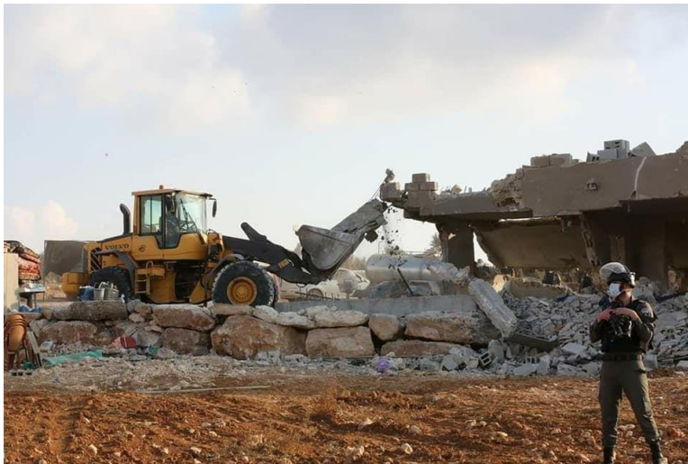
Figure 1: A home demolished in Yatta, Hebron, November 2020
