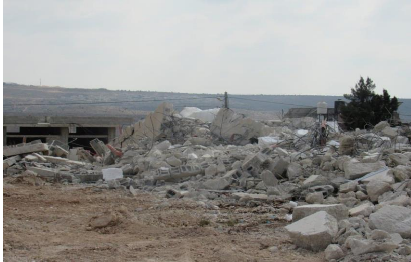
Figure 3: A wedding hall demolished in Khirbet Jubara, Tulkarem, September 2020
